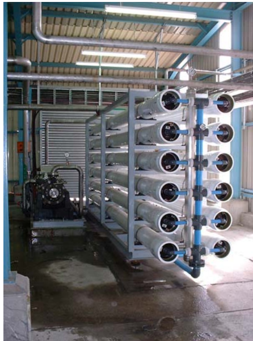
Turnkey water recycling plant customized to Clients wastewater needs at a Steel Mill.
